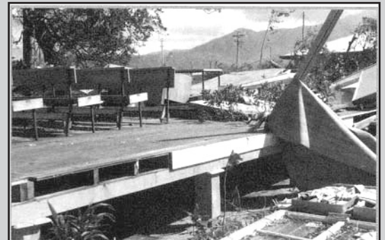
Damage from Cyclone Yasi in Queensland
